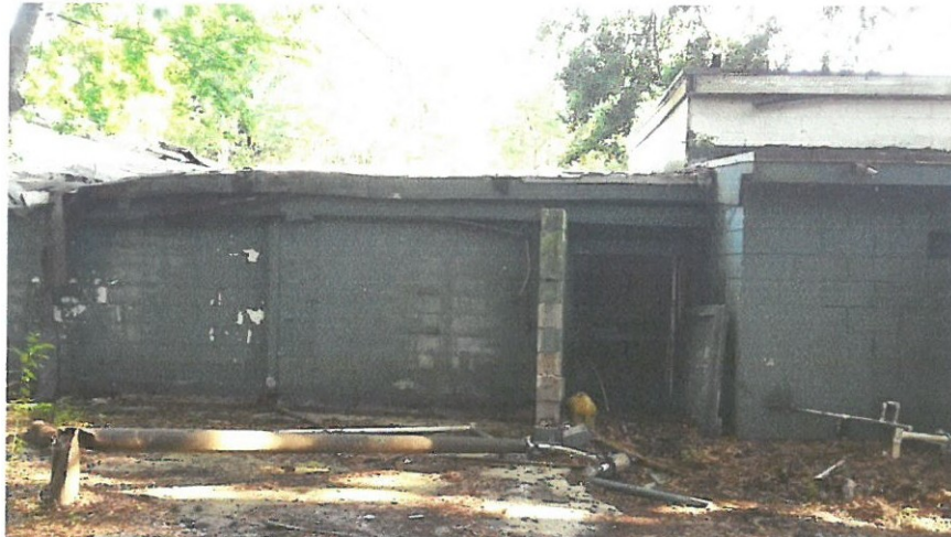
Photo 5 - Rear center of building. Note opening to interior and damaged roof section at left.
