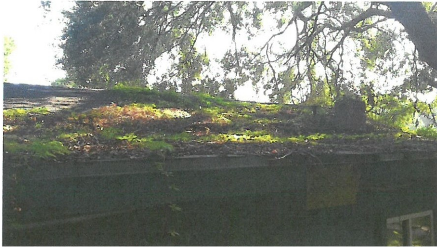
Photo 1 - Overhanging tree at east end of building over the Fish Market space. Much debris and lack of maintenance has caused this roof to fail allowing rainwater to enter.
