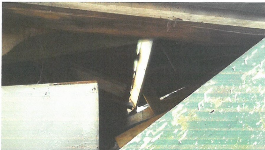
Photo 3 - Collapse of roof structure near center of building, as seen from rear window.
