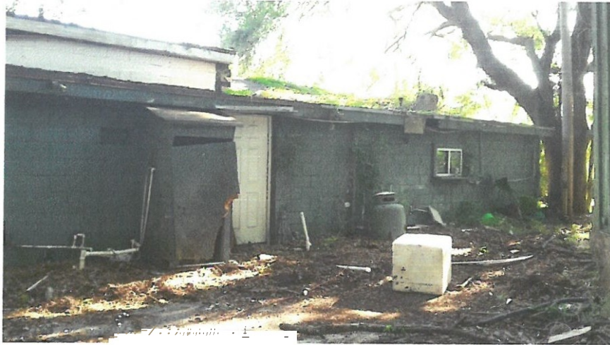
Photo 4 - East side of rear of building, behind the Fish Market and the Dress Shop. Note damaged roof fascia over window.
