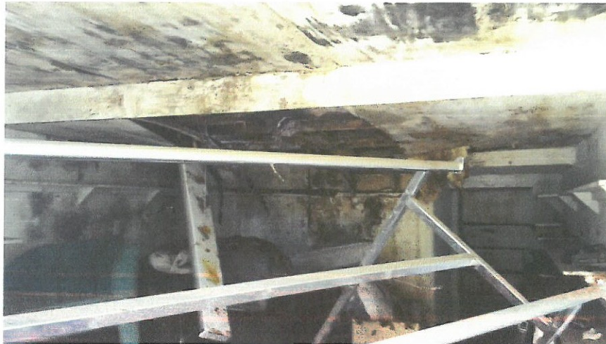
Photo 2 - Interior structural damage of ceiling/roof system near center portion of the building.
