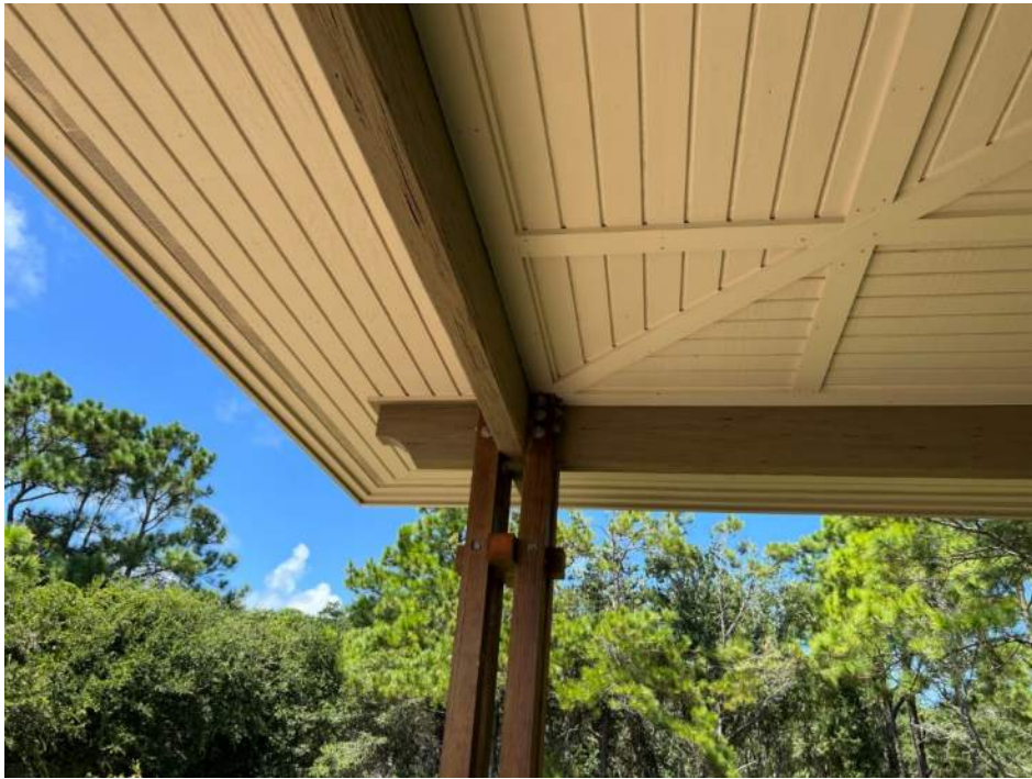
Stained columns, painted beams and ceiling.
