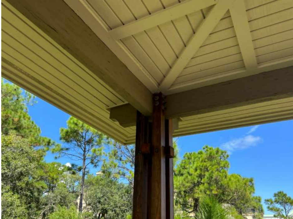
Stained columns, painted beams and ceiling.
