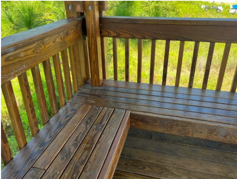
Stained bench, railing, columns.
