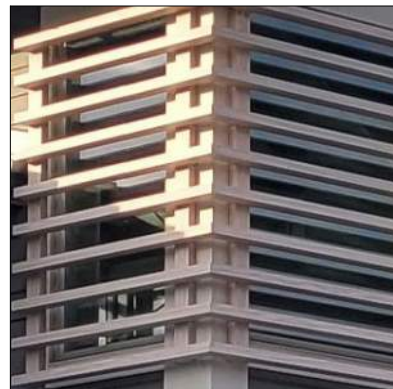
WD-01 NEW WOOD COLUMN / BEAMS, FASCIA AND LOUVERS / T&G CEILING WOOD SPECIE: SOUTHERN YELLOW PINE - SMOOTH FINISH PENETRATING SEMI- TRANSPARENT STAIN & SEALER SAMPLE COLOR: VALSPER - MONTICELLO TAN
