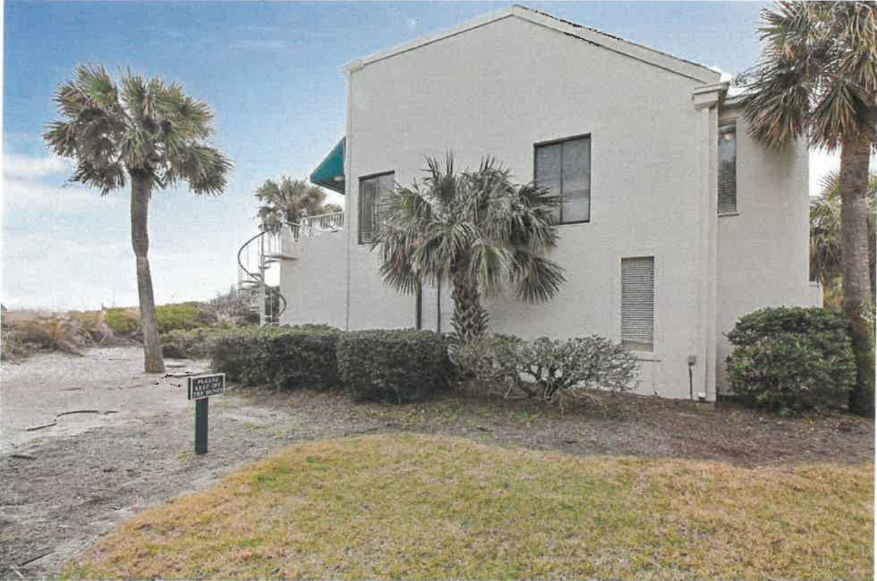
Side View showing flat roof on beach side with sloped shingle roof on street side.
