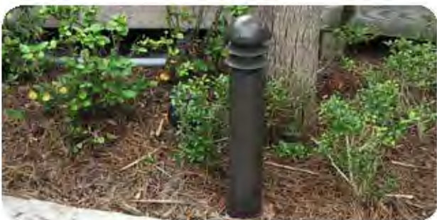
Existing Pathway Bollard Light
