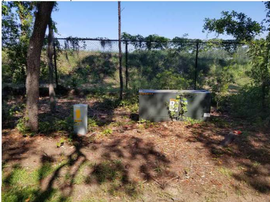
Existing Transformer, No planting within 10' (JKT 06/01/2018)
